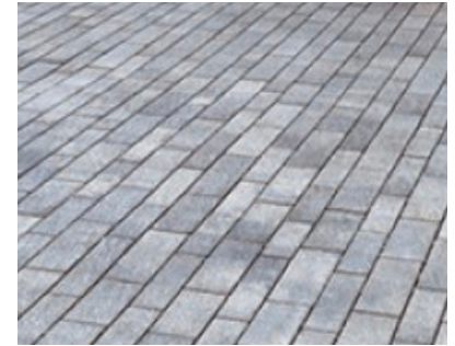
Unilock Eco-Line pavers in "Smooth-Natural" at internal pedestrian paths and garage entry
